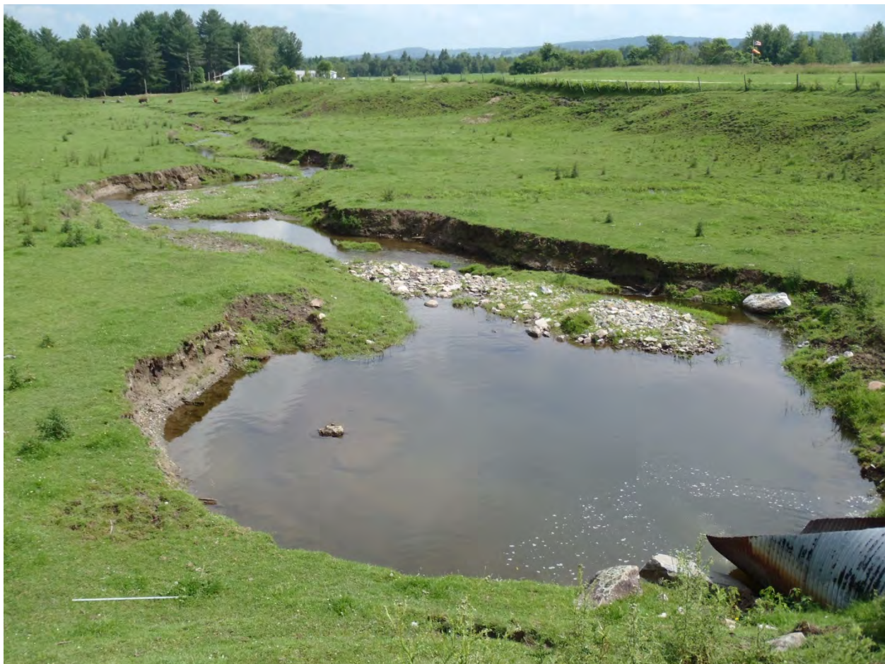
Figure 7. A large scour pool has formed at the outlet of an undersized culvert. Additionally, animals are grazed in this pasture and have direct access to the stream.
