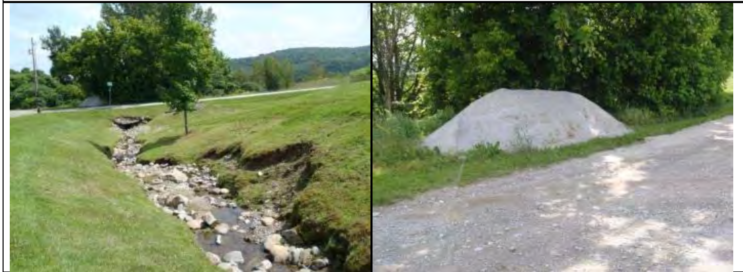
Photo 1. Ditch bank slumping Photo 2. Gravel pile directly above culvert
