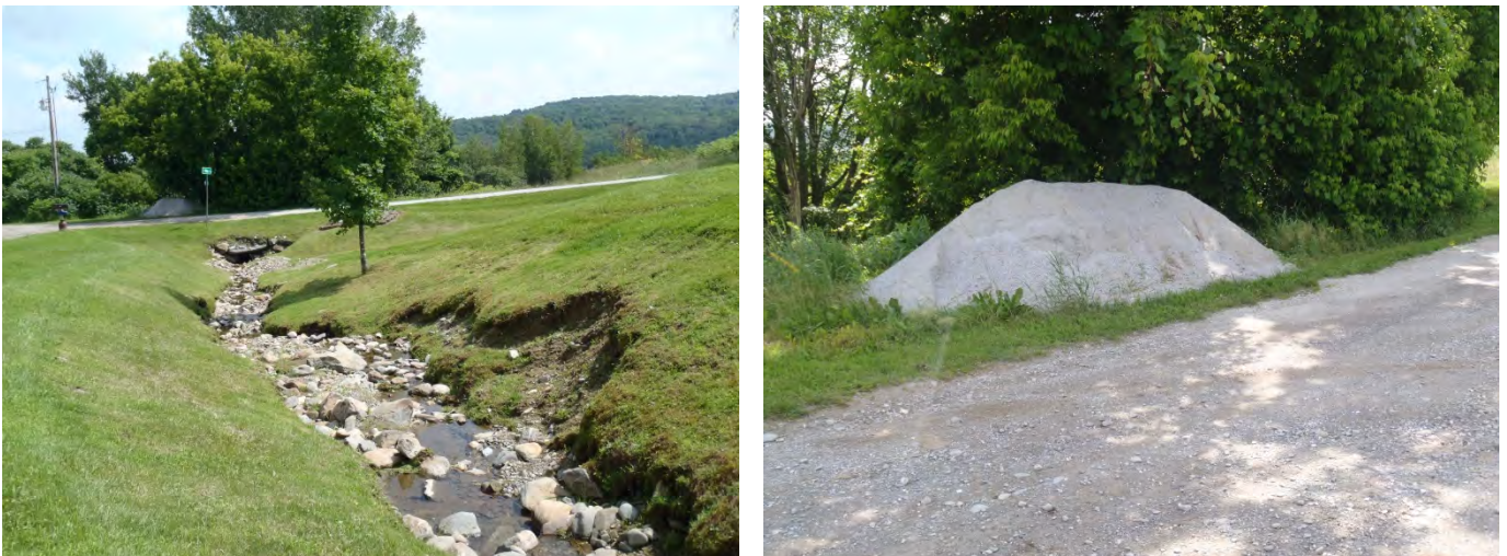
Figure 4. At left, eroding stream banks are sloughing into the stream. Vegetation is mowed up to the edge of the banks. At right, a large gravel stockpile sits 10 feet from the stream.
