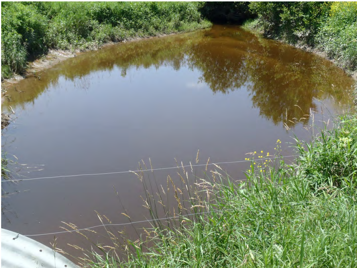
Figure 9. A large scour pool immediately downstream from the undersized culvert beneath Bushey Road.
