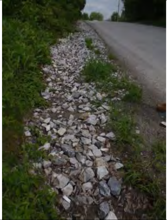
Photo 10. Rock-lined ditch, sediment choked
