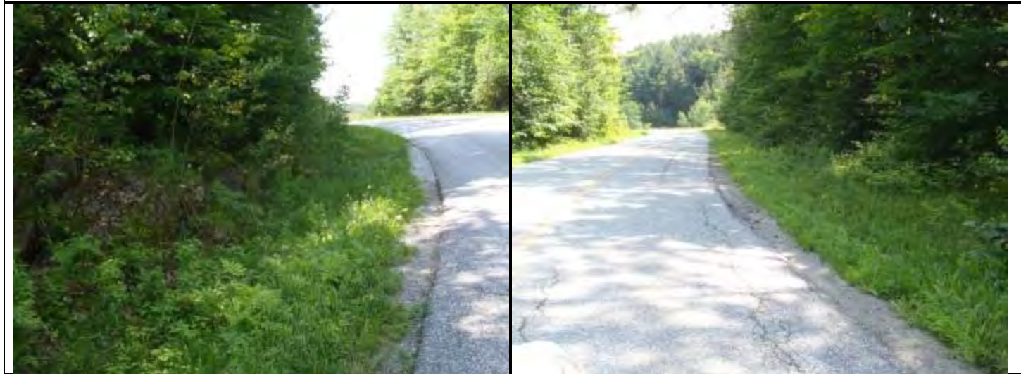
Photo 1. Erosion at edge of road Photo 2. Erosion at edge of road
