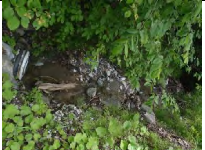
Photo 4. Sediment deposited in ditch
