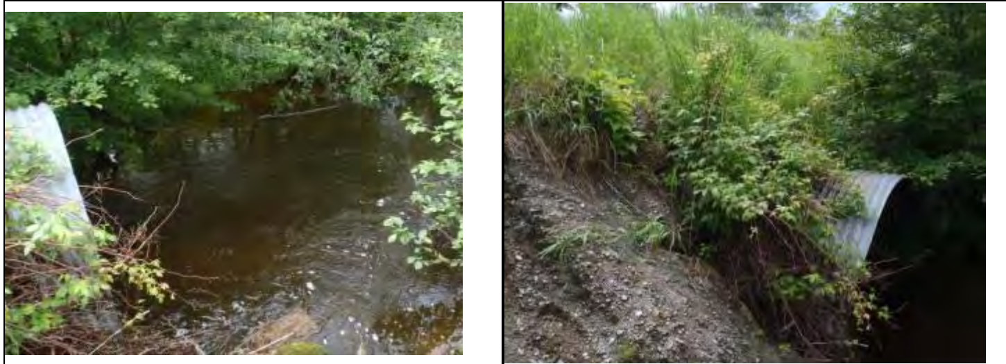
Photo 1. Scour pool Photo 2. Bank erosion around culvert
