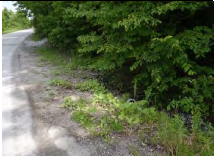
Photo 6 Ditch bank collapse and sediment deposit
