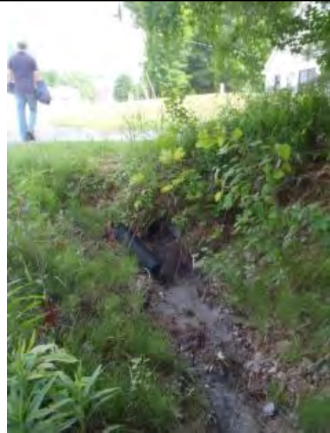
Photo 20. Sediment deposited at a culvert outfall
