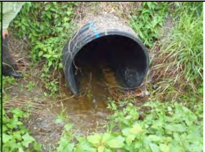
Photo 2. Stream bed is eroded 2 inches below invert of culvert inlet.
