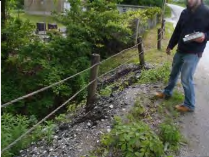
Photo 3 Shoulder above culvert inlet
