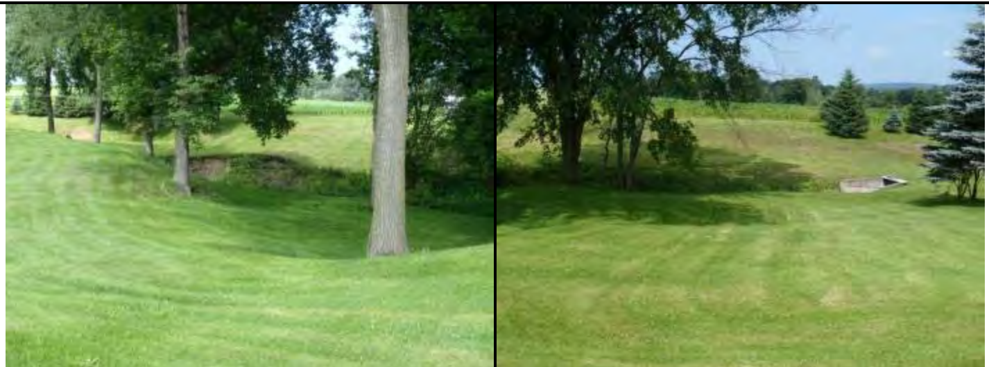
Photo 1. Eroded stream bank downstream from culvert
